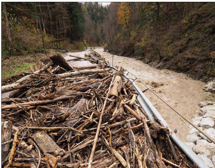
Slika 7: Zasuti cestni propusti (foto: P. Rotar) Figure 7: Blocked road culverts (Photo: P. Rotar)
