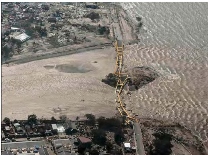
Slika 5: Porušen most Kuning Ponulele (vir: https://www.reuters.com/news/picture/earthquake-and-tsunami-devastate-indonesidUSRTS23EU8 )
