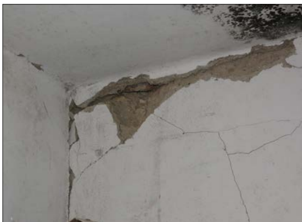
Slika 10: Široke in globoke razpoke nosilnega zidu na Vinjem Vrh (foto M. Godec) Figure 10: Large and extensive cracks in bearing wall in Vinji Vrh (Photo M. Godec).
