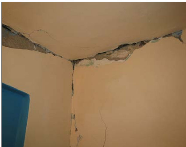
Slika 6: Široke in globoke razpoke na stikih nosilnih zidov in stropa na Stojanskem Vrh (foto M. Godec) Figure 6: Large and extensive cracks in the joints of walls and ceiling in Stojanski Vrh (Photo M. Godec).
