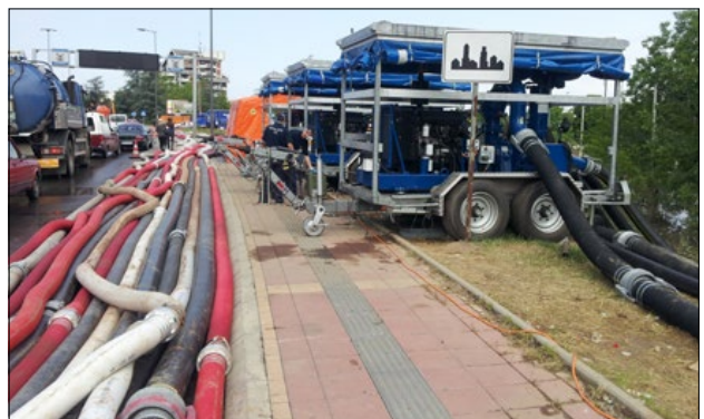
Slika 6: Tri visoko zmogljive črpalke DIA AVS so sodelovale pri prečrpavanju vode v mestu Obrenovac. (foto: J. Melanšek) Figure 6: Three high-capacity DIA AVS pumps were used for water pumping in the town of Obrenovac. (photo: J. Melanšek)
