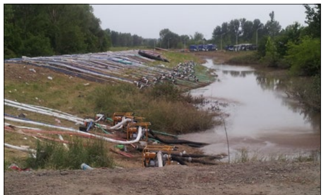
Slika 8: Srbske gasilske enote prečrpavajo vodo prek nasipa reke Kolubare. (foto: E. Pogačar) Figure 8: Serbian fire units pumping the water over the Kolubara river dike. (photo: E. Pogačar)
