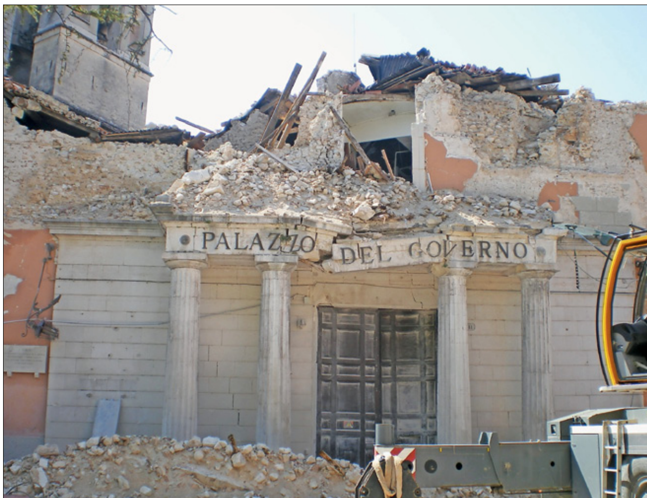
Slika 2: Lokalna prefektura v L'Aquila je bila ob potresu močno poškodovana. Figure 2: The local prefecture in L'Aquila is heavily damaged by the earthquake.
