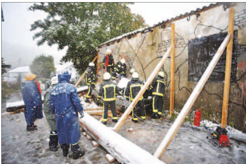
Slika 5: Aktivnosti USAR in podpiranje poškodovanega objekta Figure 5: USAR operations – propping up of a damaged facility.
