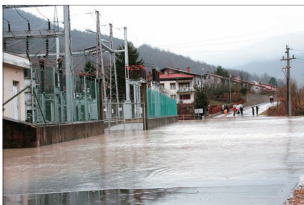
Slika 6: RTP v Plavah (25. decembra 2009 ob 12. uri) (foto: M. Kogoj) Figure 6: The Plave Substation (25 December 2009 at noon) (photo: M. Kogoj)
