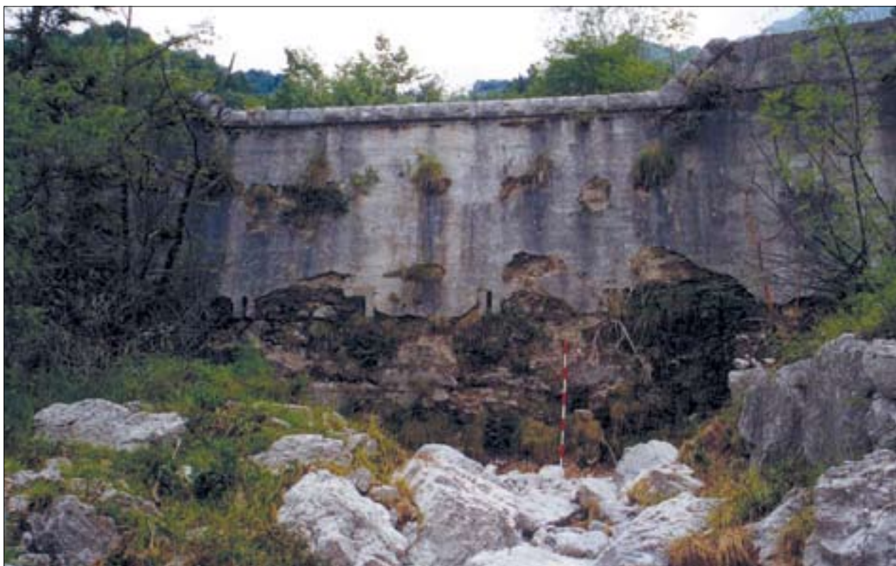
Slika 5. Poškodovana betonska pregrada (hudournik Prekopa) Figure 5. Damaged concrete dam (Prekopa Flood)
