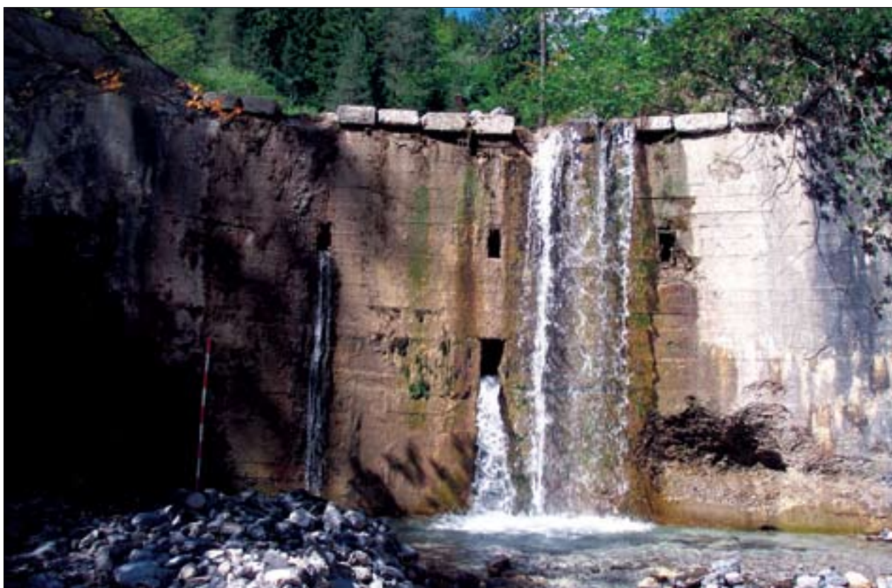
Slika 7. Poškodovana betonska pregrada (hudournik Belca) Figure 7. Damaged concrete dam (Belca Flood)
