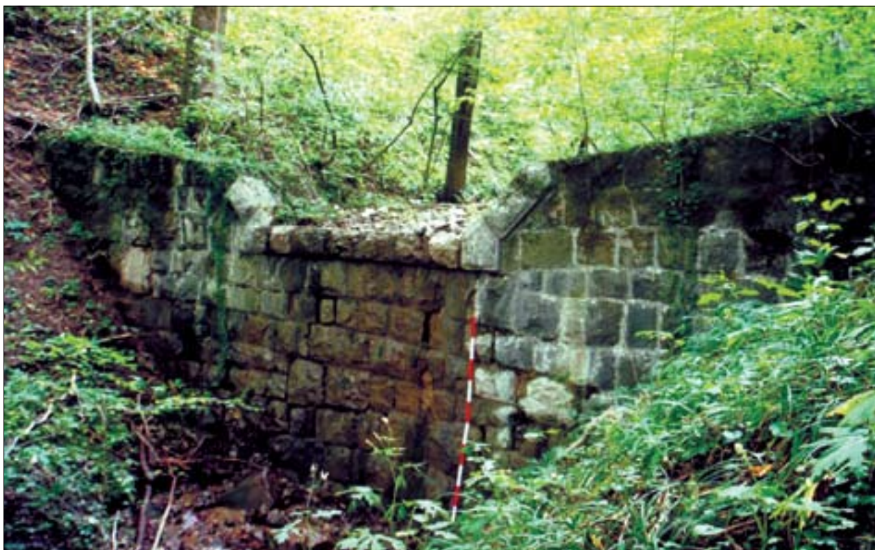
Slika 2. Več kakor 80 let stara hudourniška pregrada, zidana v cementni malti (hudournik Kred) Figure 2. 80-year-old dam in stone masonry (Kred Flood)
