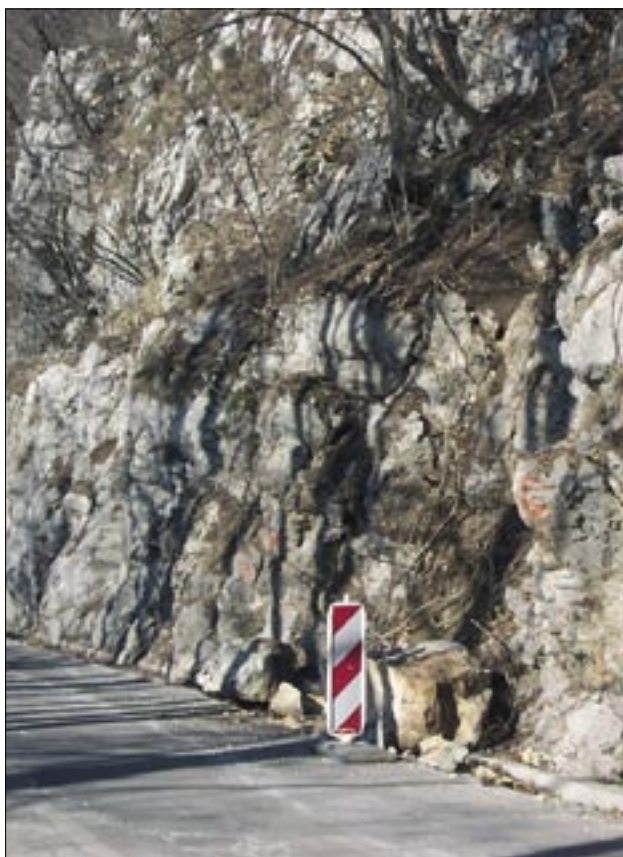
Slika 1. Ostanke skal na regionalni cesti pri Colu po poružitvi dne 04. 02. 2006 (foto: T. Jeršič) Figure 1. Rocks on the regional road near Col after a rockfall on 4 February 2006 (photo: T. Jeršič)
