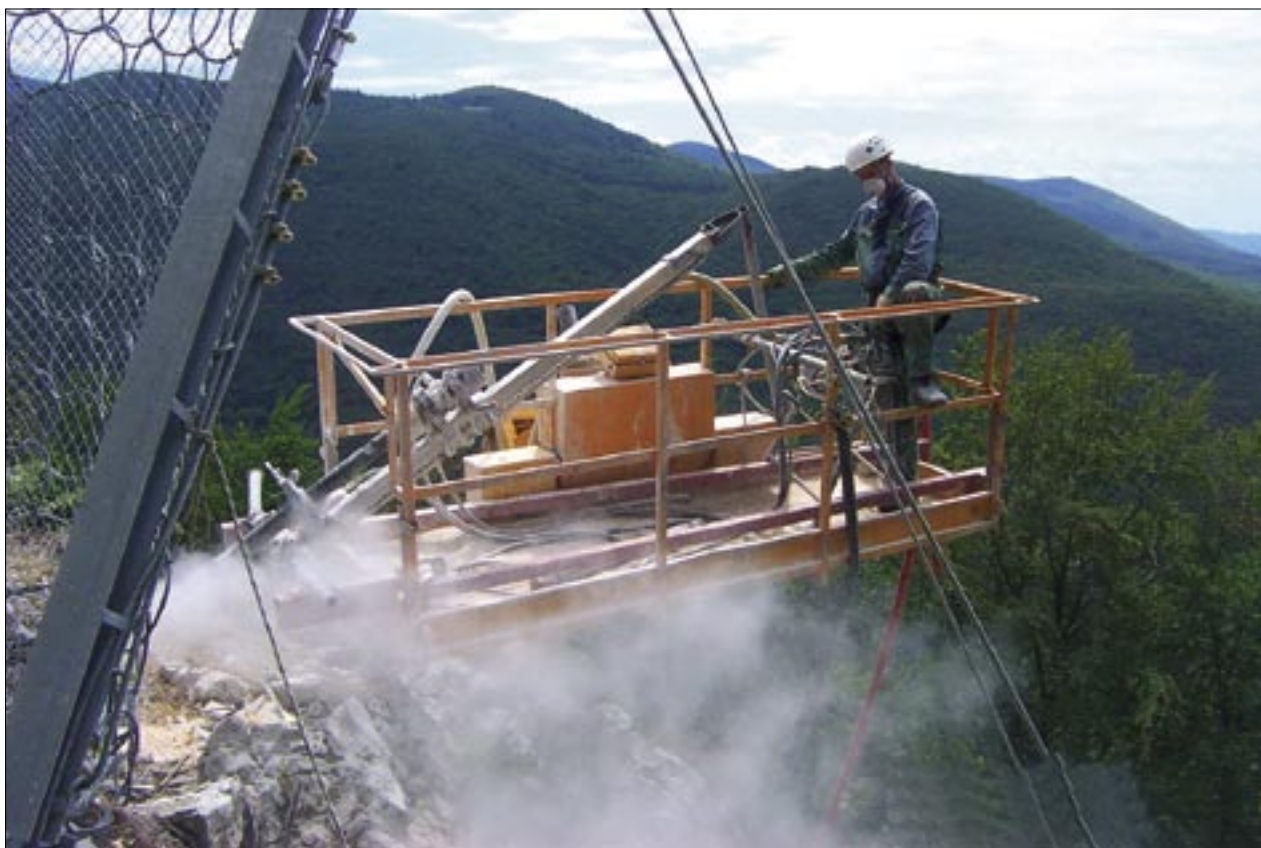
Slika 6. Vrtanje lukenj za sidra s prenosno vrtno garnituro, s pomočjo avtodvigala (foto: A. Rus) Figure 6. Drilling anchor holes using a portable drilling set with the help of a car jack (photo: A. Rus)
