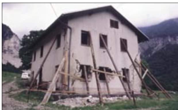
Slika 11. Ob potresih 1998 in 2004 v Posočju so bili številni objekti domnevno bolj poškodovani zaradi resonančnih učinkov med sedimenti in zgradbami. Figure 11. In the 1998 and 2004 earthquakes in the Upper Soča valley several buildings were presumably damaged more because of resonance effects between sediments and structures.
