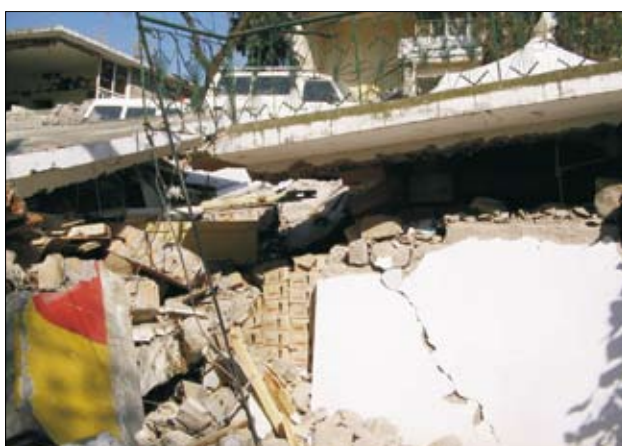
Slika 10. Potres ni prizanesel niti skladiščem zdravil Figure 10. The earthquake didn't even spare a medicine storehouse.
