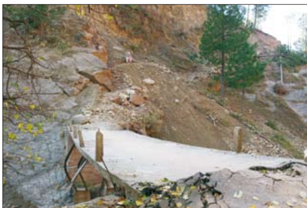
Slika 9. Tukaj je bila pred potresom cesta. Zdaj pa... Figure 9. There was a road here before the earthquake. Now ....
