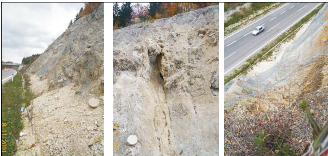
Slike 10, 11 in 12. Polica 7L – stanje pred ukrepanjem – velika prometna ogroženost Figures 10, 11 and 12. Polica 7L – situation before measures – major traffic hazard
