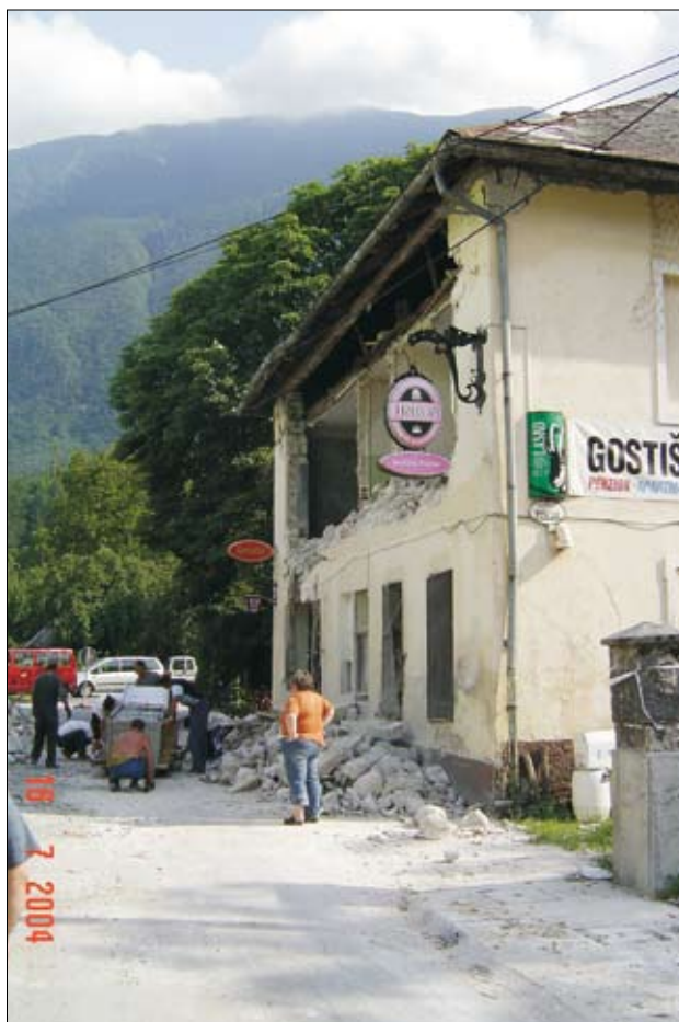
Figure 2. Number of buildings damaged during 2004 earthquake and a damaged building (grade 5) in Čezsoča.
