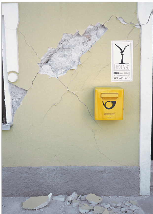
Slika 8. Diagonalne razpoke na pošti v Čezsoči Figure 8. Diagonal crack on the post office in Čezsoča
