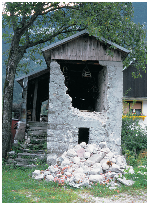
Slika 19. Uničena zgradba v vasi Čezsoča Figure 19. Destroyed building in the village of Čezsoča
