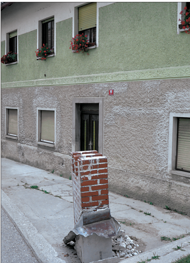
Slika 5. Najpogostejše poškodbe so bili poškodovani ali odpadli dimniki, ki so jih zaradi nevarnosti nadaljnjih poškodb že takoj po potresu odstranjevali gasilci. Figure 5. The commonest damage was damaged or falling chimneys, which firefighters removed immediately after the earthquake because of the danger of further damage.
