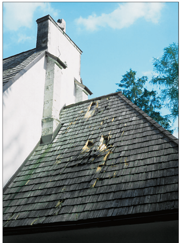
Slika 6. Ponekod so odpadli dimniki poškodovali strešno kritino. Na sliki je poškodovana cerkev pri kampu v Bovcu, kjer je odpadli zvon poškodoval strešno kritino. Figure 6. In places falling chimneys damaged roof coverings. The picture shows the damaged church by the camp in Bovec, where a falling bell damaged the roof covering.
