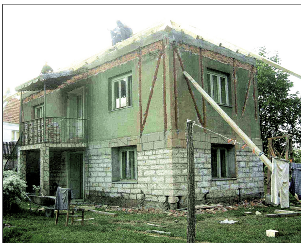
Slika 2. Primer po sistemu DC90 potresno ojačanega objekta v Mionici Figure 2. Mionica - an example of an earthquake-braced structure in accordance with the DC90 system
