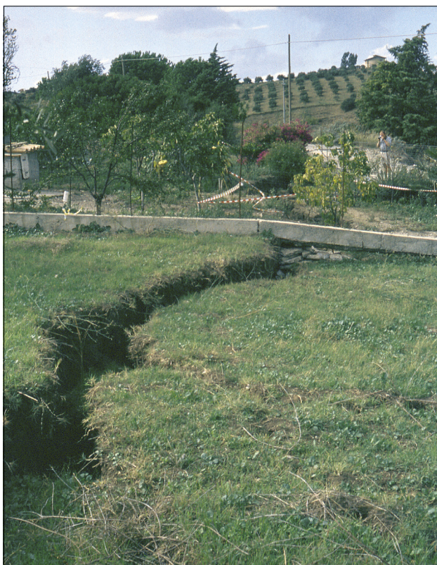
Figure 4. A detailed snapshot of the direction of the landslide direction. On the road near the well, a fissure occurred and the bridge moved.
