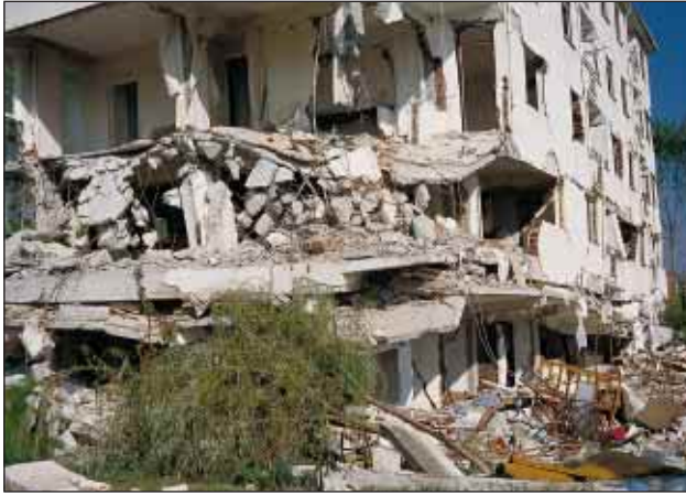
Slika 4. V turškem potresu uničen stanovanjski blok v Seymenu. (foto: R. Vidrih) Figure 4. A residential block of flats in the city of Seymen was destroyed in the Turkey earthquake (photo: R. Vidrih)
