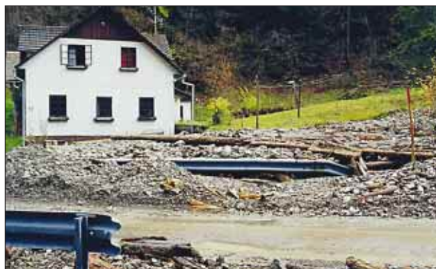
Slika 9. Ogrožena stanovanjska hiša ob hudourniku Poličnikov potok (foto: T. Jeršič) Figure 9. A residential building located alongside the Poličnikov torrent (photo: T. Jeršič)
