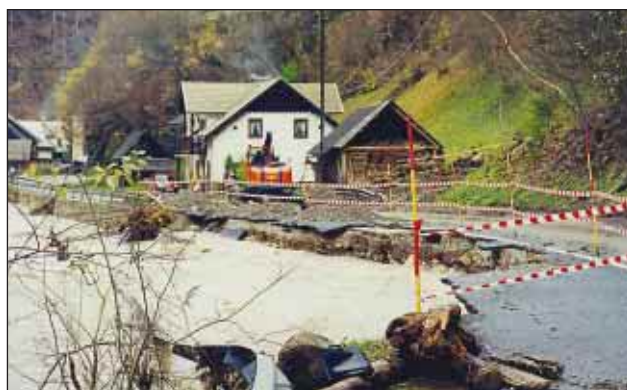
Slika 8. Posledice, ki jih zaradi neustreznih ali dotrajanih obrežnih zavarovanj lahko utrpijo cestne prometnice, so pogosto katastrofalne. (foto: T. Jeršič) Figure 8. The consequences suffered by roads due to inadequate or deteriorated protective measures are often catastrophic (photo: T. Jeršič)
