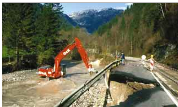
Slika 6. Interventni ukrepi za preprečevanje nadaljnega zaježanja s preusmeritvijo glavnega toka vode in izvedbo začasnega bočnega zavarovanja. (foto: J. Papež) Figure 6. Intervention measures aimed at preventing further lateral erosion by means of deviation of the main stream as well as the construction of a temporary protection (photo: J. Papež)
