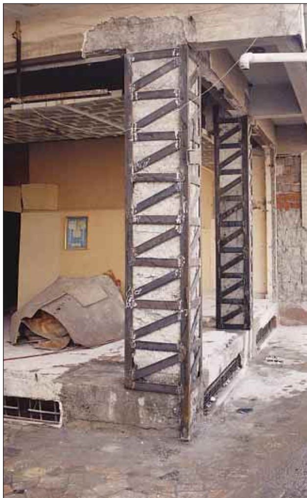
Slika 13. Takoj po potresu so začeli ne le z odstranjevanjem ruševin, ampak tudi z ojačevanjem. Primer na sliki kaže ojačevanje poškodovanih stebrov. (foto: M. Godec) Figure 13. Immediately after the earthquake, people not only began to remove the ruins, but also to reinforce the buildings. The photo shows the reinforcement of damaged pillars. (photo: M. Godec)
