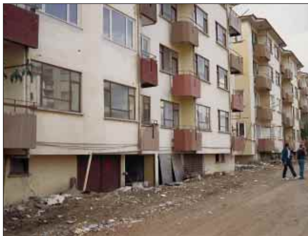
Slika 15. Posedanje objektov zaradi slabih geoloških razmer. (foto: R. Vidrih) Figure 15. Subsidence of buildings due to unfavourable geological conditions. (photo: R. Vidrih)
