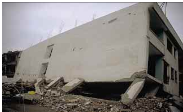
Slika 4. Mehko pritličje s šibkimi stebri v prečni smeri (foto: M. Fisching) Figure 4. Soft first story with weak columns in the transverse direction (photo: M. Fisching)
