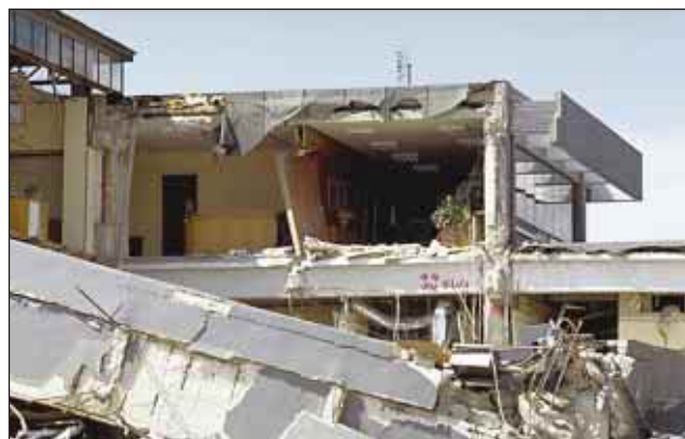
Slika 6. Detajl porušene tovarne Figure 6. Detail of collapsed factory
