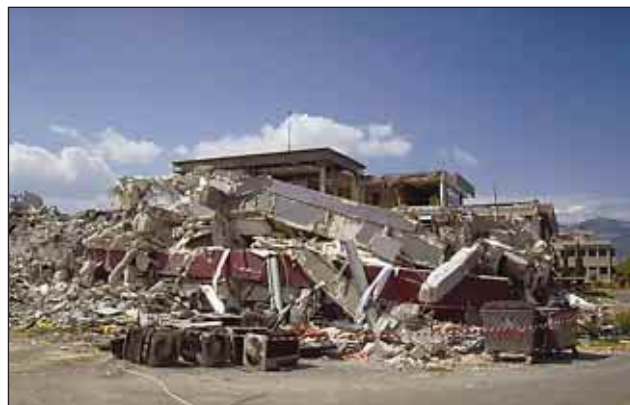
Slika 5. V večjem delu tovarne »Fourlies« so bile težko poškodovane konstrukcije Figure 5. Part of the »Fourlies« factory building collapsed and the remainder suffered serious structural damage
