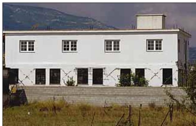
Slika 7. Mnoge poškodbe objektov vzdolž ulice Dekelias v Atenah Figure 7. Several damaged buildings along Dekelias Road (Athens)
