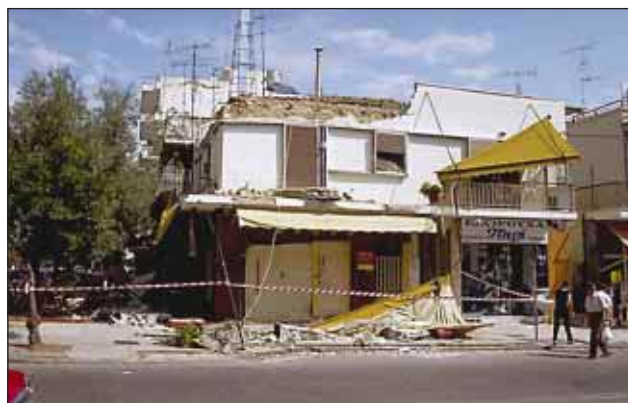
Slika 3. Težke poškodbe objektov vzdolž ulice Dekelias Odos v Atenah Figure 3. Heavily damaged building along Dekelias Odos Street (Athens)
