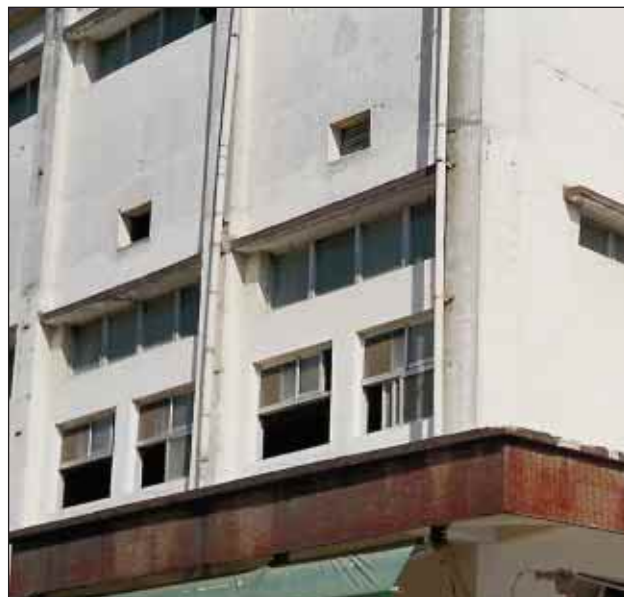
Slika 5. Vzrok porušitve industrijskega objekta je bila mehka etaža (foto: R. Vidrih) Figure 5. The reason for the collapse of the industrial building was soft storey (photo: R. Vidrih)
