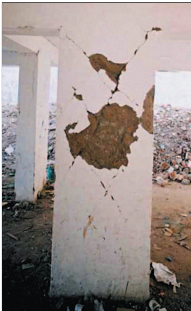
Slika 7. Strižna porušitev stebra v pritličju stanovanjske hiše Figure 7. Shear failure of column on the ground floor of the building.
