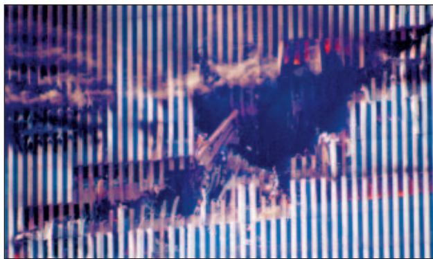
Slika 8. Poškodbe zunanjih stebrov zaradi udarca v severno fasado WTC 1 (foto: R. Rabanne) Figure 8. Impact damage to exterior columns of the north face of WTC 1 (photo: R. Rabanne)
