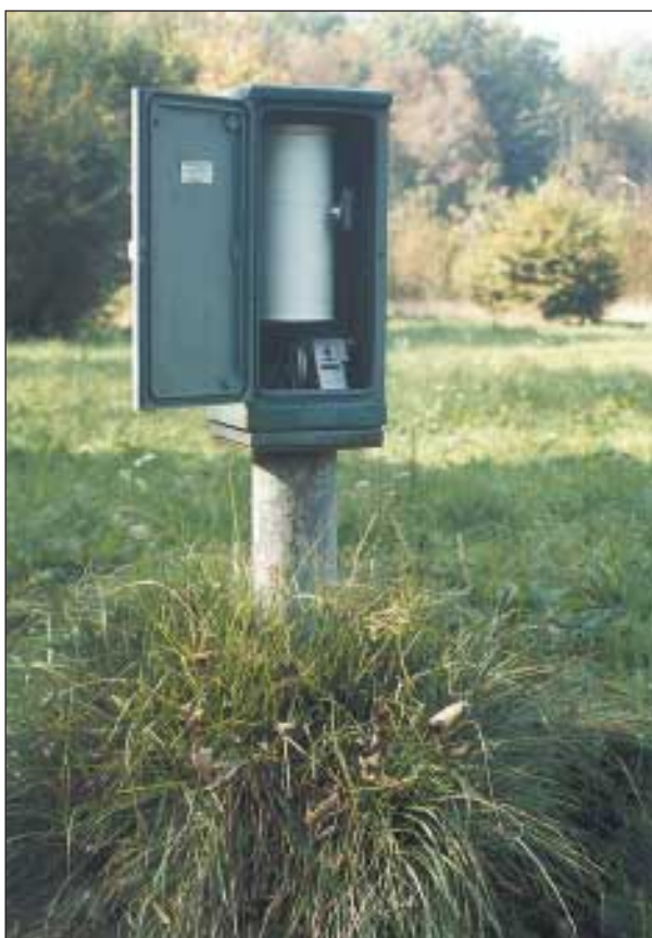
Slika 2. Merilno mesto višine gladine podzemne vode S-3667 Drulovka (arhiv HMZ) Figure 2. Groundwater level observation station S-3667 Drulovka (courtesy of HMZ)
