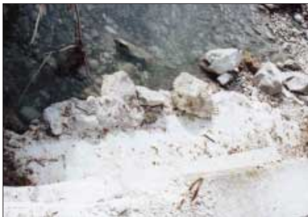
Slika 9. Majhni lomljeni kamni, ki so jih uporabili za kameni zamet; take je voda odkotalila po strugi navzdol; »kameni zameti« so izginili; zaščite temeljev ni bilo več (foto: S. Trček) Figure 9. The stones used for the protective barrier were too small in size, and were consequently carried downstream by rushing waters. The "stone barrier" has disappeared and the foundations exposed to the power of water (photo: S. Trček)
