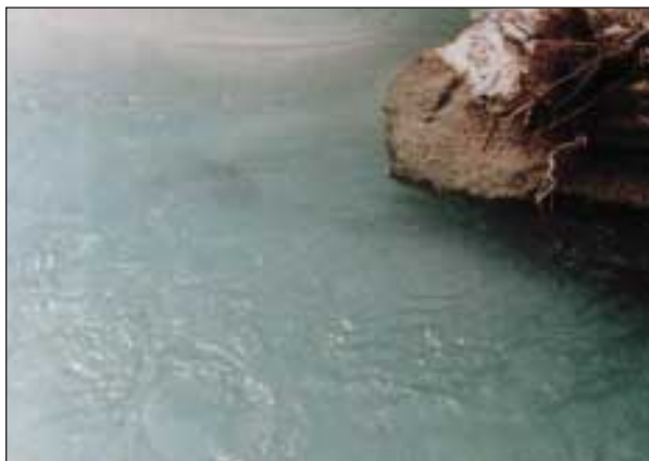
Slika 11. Spodjeden betoniran »kameni zamet« na dolvodni strani poseđenega podpornika (foto: S. Trček) Figure 11. The base of a concreted "stone barrier" on the downstream side of a sunken support has been washed away. (photo: S. Trček)
