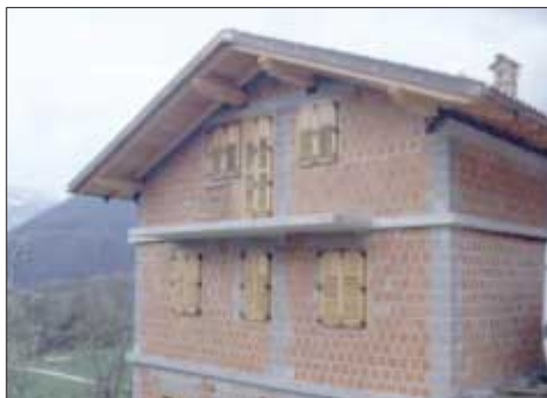
Slika 3. Ustrezno zgrajena zidana hiša, nepoškodovana med potresom v Posočju leta 1998 (foto: Matej Fischinger) Figure 3. Properly constructed masonry building, undamaged during the Bovec 1998 earthquake (photo: Matej Fischinger)
