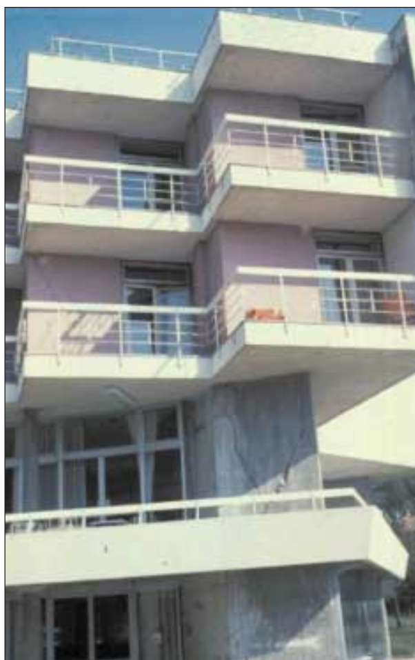
Slika 6. Poškodbe naknadno zgrajene stene hotela v Petrovcu na moru (foto: P. Fajfar) Figure 6. Damaged wall of a hotel in Petrovac, built during repair and strengthening of the structure (photo: P. Fajfar)
