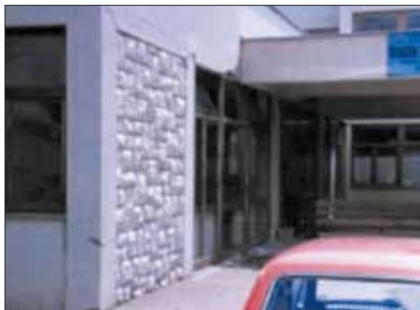
Slika 5. Poškodovana konstrukcija zdravstvenega doma v Ulcinju (foto: P. Fajfar) Figure 5. Damaged structure of the Municipal Health Centre in Ulcinj (photo: P. Fajfar)
