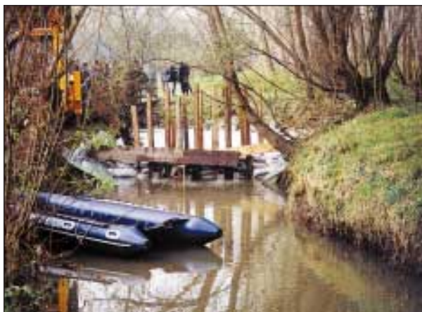
Slika 9. Pripadniki oddelka za tehnično reševanje MO Murska Sobota in VGP Mura so postavili t. i. sifonsko pregrado na rokavu Mure. (foto: S. Jauk) Figure 9. Members of the Technical Rescue Department of MO Murska Sobota and VGP Mura setting up the siphon barrier in a branch of the Mura River. (photo: S. Jauk)
