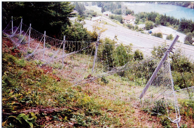
Slika 7. Drča III – zaključek del (foto: D. Durjava) Figure 7. Chute III - completed works (photo: D. Durjava)
