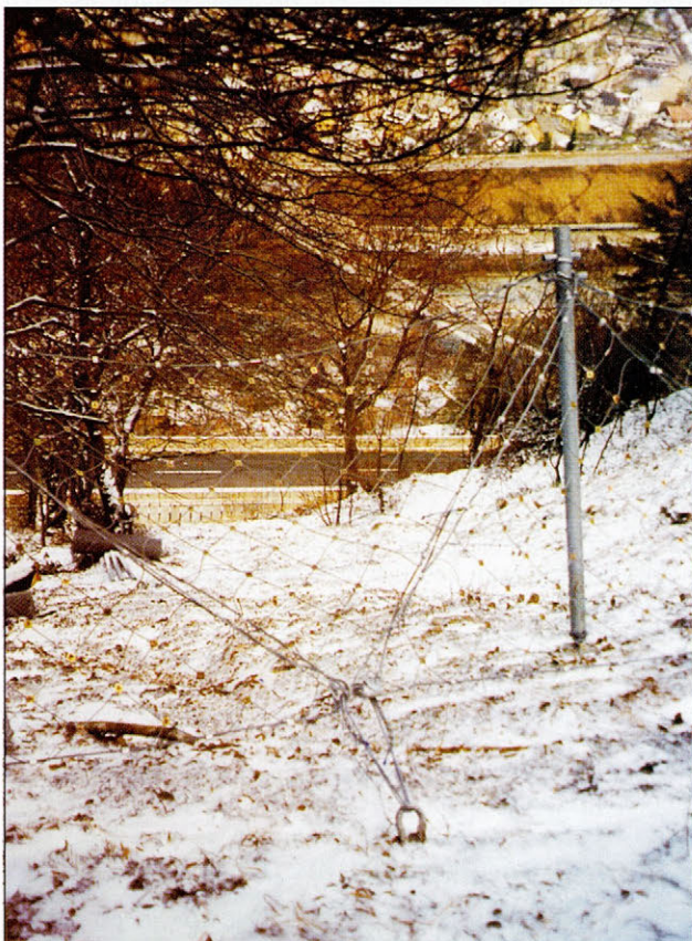
Slika 2. Drča III – montaža pod skokom (foto: D. Durjava) Figure 2. Installation works below step (photo: D. Durjava)
