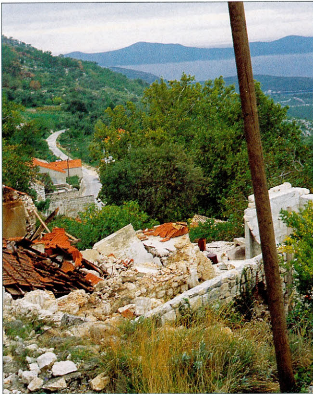
Slika 2. Večina slabo zgrajenih hiš v dubrovniškem primorju, predvsem vseh Mravinca, Podimoč in Trnava, je bilo ob potresnih sunkih porušeni (foto: R. Vidrih) Figure 2. Most of the poorly built houses in the Dubrovnik littoral region, especially in the villages of Mravinca, Podimoč and Trnava, collapsed during the earthquake (photo: R. Vidrih)
