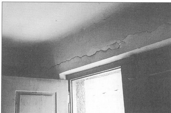
Slika 3. Razpoke v ometu gasilskega doma v Ilirski Bistrici, Titov trg 11 (foto: R. Vidrih) Figure 3. The cracks in the plaster at the fire-station in Ilirska Bistrica, Titov trg 11 (photo: R. Vidrih)
