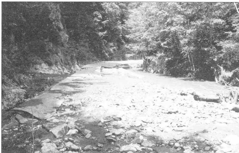
Slika 1. Kotredešica v soteski Tesen – voda je uničila asfaltno cesto in spodjedla podporne zidove Figure 1. The Kotredešica in the narrow valley Tesen – demolished asphalt road and retaining walls
