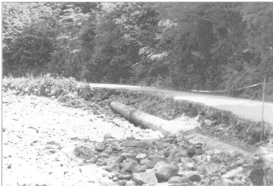
Slika 6. Hudournik Mislinja nad Mislinjo: Neutrjene brežine ceste, prekopane zaradi polaganja cevovoda za MHE Glinšek, so hitro popustile pred utesnjenimi hudournimi vodami Mislinje. Foto: Zoran Fujs Figure 6. Torrential stream Mislinja at Mislinja: The Mislinja easily carried off most of a road already partially ripped up in order to lay down a waterline. Photo: Zoran Fujs
