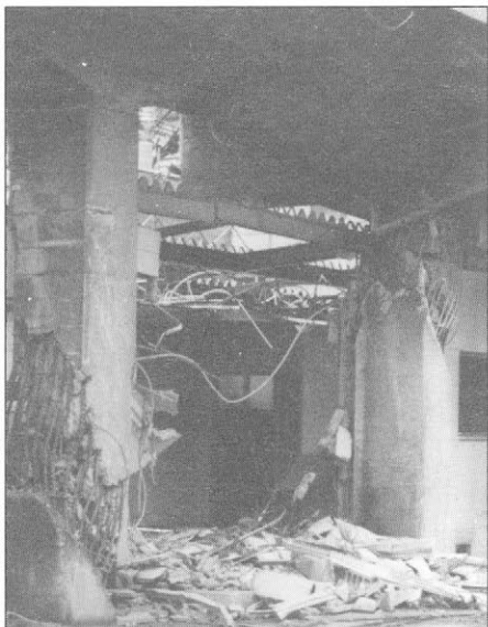
Slika 10. Težko poškodovani stebri nadvoza železniške proge Hankyu Railway Figure 10. Heavily damaged columns of the elevated Hankyu Railway
