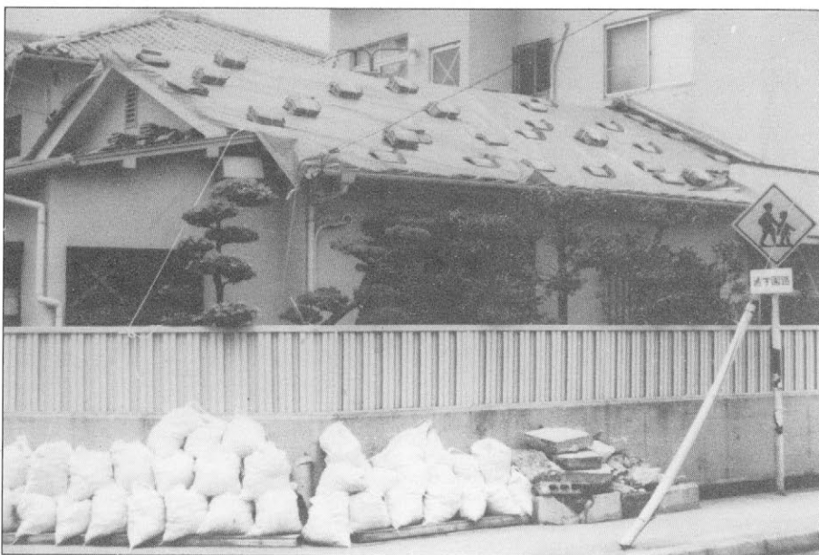
Slika 6. Prebivalci so strehe zaradi poškodovane kritine sami prekrili s polivinilskimi ponjavami, ki so jim jih po potresu razdelile mestne oblasti Figure 6. People covered their houses with polyethylene sheets provided by city authorities
