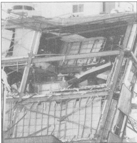
Slika 16. Potrgane diagonale in poškodbe vozlišč Figure 16. Broken diagonal braces and damage to joints
