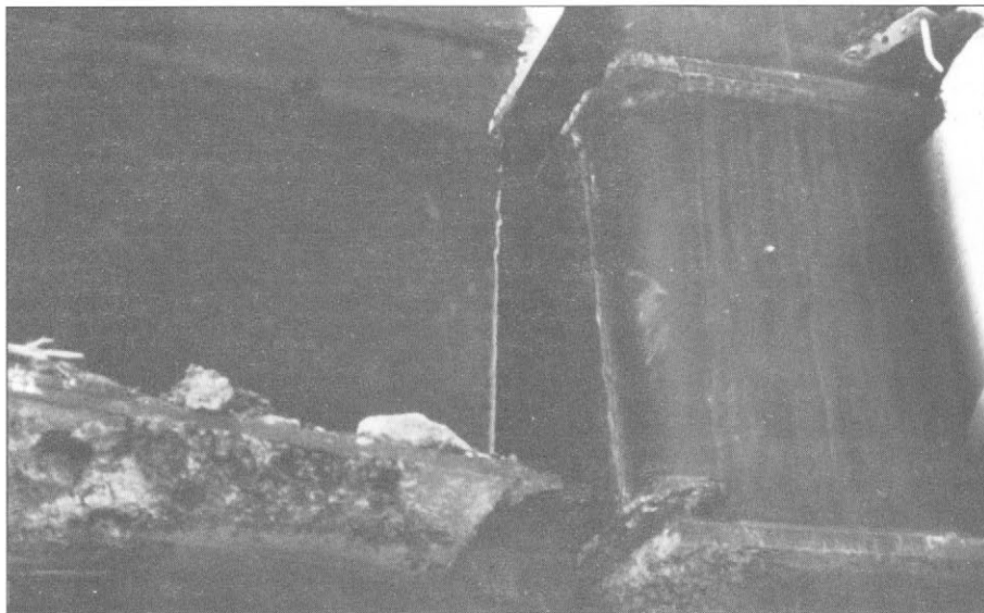
Slika 15. Porušitev zvara na stiku stebra z nosilcem Figure 15. Weld rupture at beam to column connection
