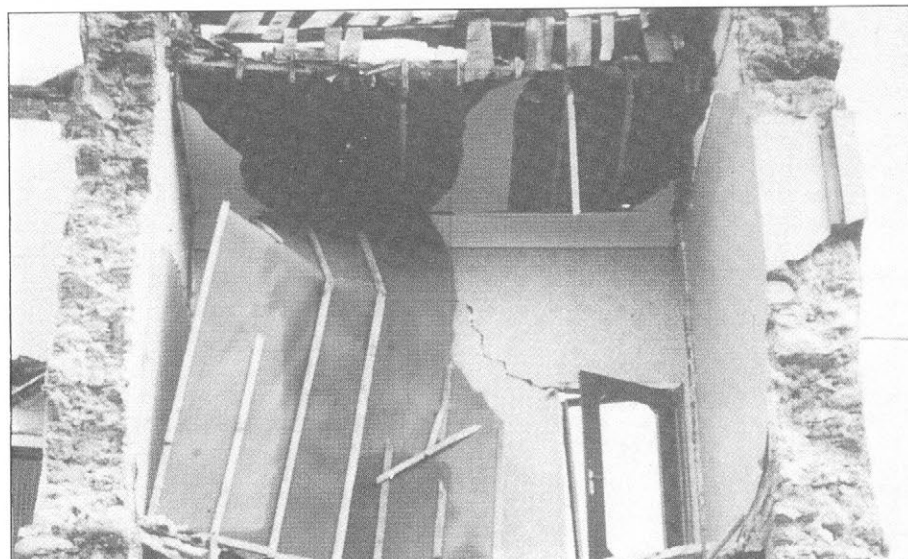
Slika 2. Potres v Italiji leta 1980 – peta stopnja poškodb (slikovni primer, ki ponazarja klasifikacijo poškodb, je sestavni del lestvice EMS-92) Figure 2. Earthquake in Batvano, Italy 1980 – damage of grade 5 (examples illustrating classifications of vulnerability and damage used in the scale EMS-92)
